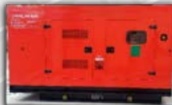
225kva 230v 3ph - San Juan City
