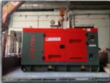
50kva 3ph 230v- San Fernando Pampanga
