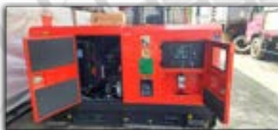
75kva 1ph 230v - Cabuyao, Laguna
