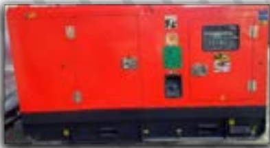
75kva 1ph 230v - Cabuyao, Laguna
