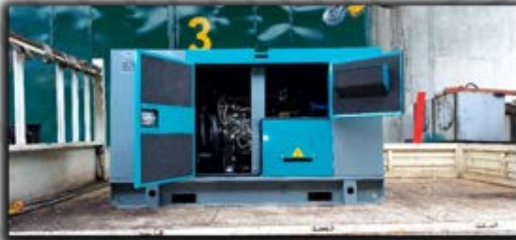
25kva 3ph 230v- Pampanga
