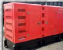
300kva 230v 3ph - Calumpit Bulacan
